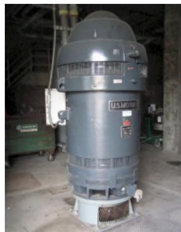
Figure 8: Example lift pump.
