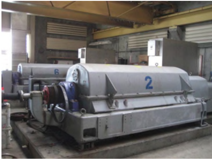
Figure 9: Example centrifuges used for sludge dewatering.
