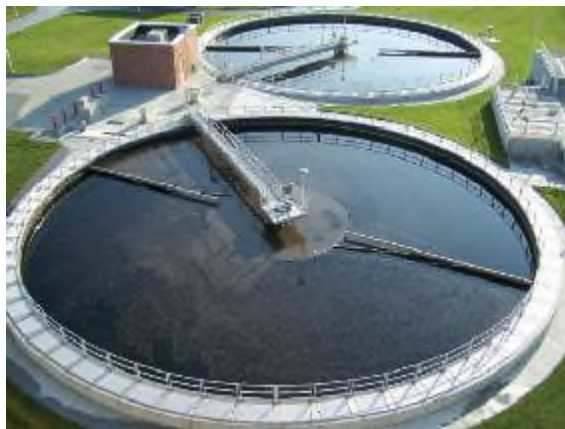
Figure 7: Example primary clarifiers.
