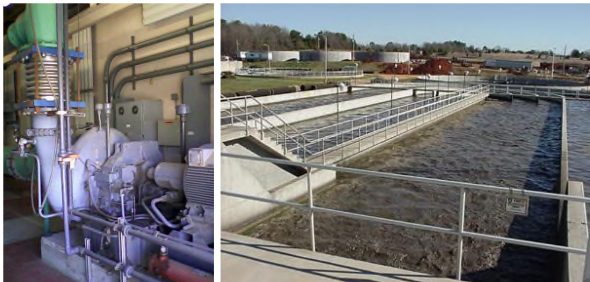
Figure 6: Blower (left) and an aeration basin (right).
